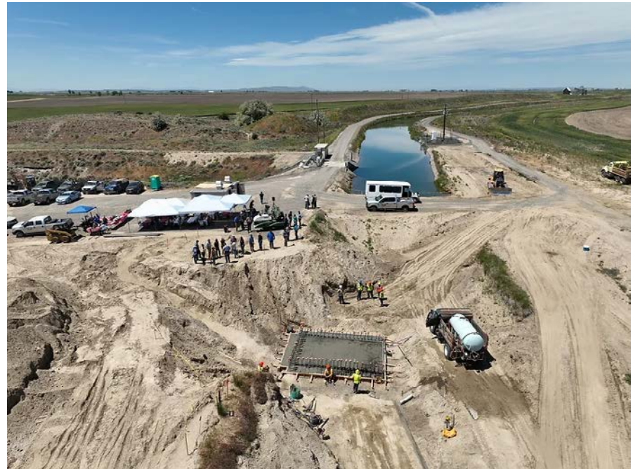
Construction at the EL 86.4 site (Courtesy of Mike Baden, Washington State Conservation Commission)
